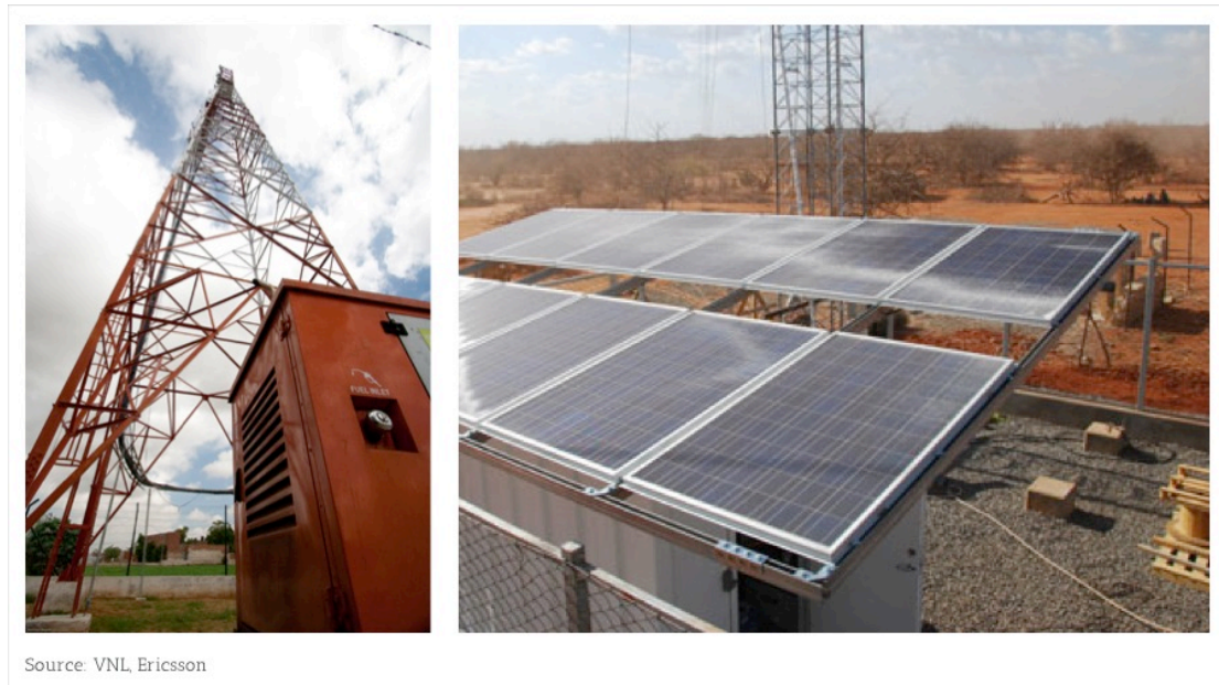
Exhibit 2 – Example of a base station powered by a diesel generator (left), and one integrating solar PV (right)
